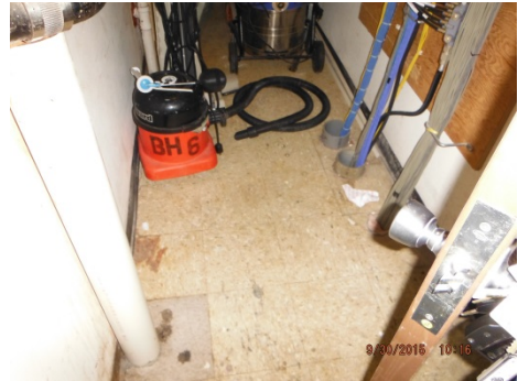
Photo 10. . Asbestos-containing tan with brown streaks 12” x 12” floor tile and associated mastic were observed in numerous locations throughout the building.
