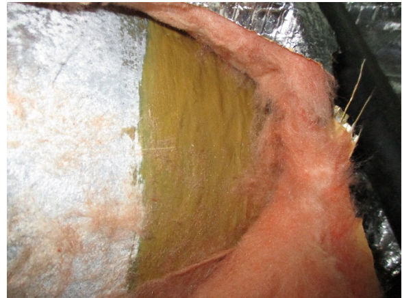
Photo 4. ACM Olive Duct Mastic under Fiberglass Insulation in 1st Floor Mechanical Room.
