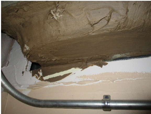
Photo 3. Non-ACM Brown Mastic on Metal Duct.
