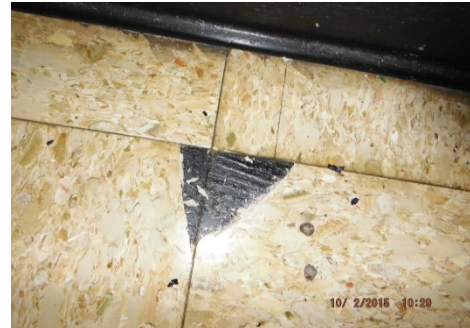
Photo 4. Asbestos-containing tan streaked 12” x 12” floor tile and associated mastic was observed in numerous locations throughout the building.
