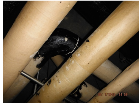
Photo 12. Asbestos-containing black mastic associated with the seams of foam glass TSI was observed throughout the building.
