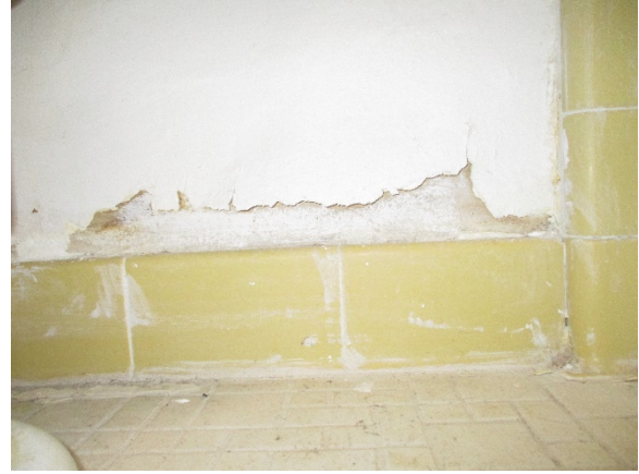
Photo 2. Damaged ACM Drywall in Room 1101.
