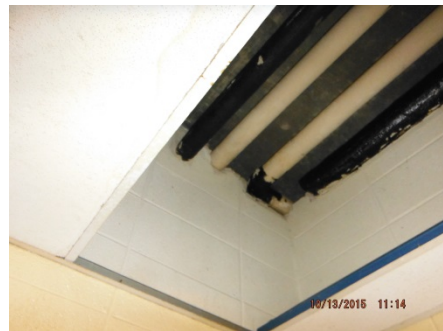
Photo 7. Asbestos-containing black mastic on fiberglass elbows was observed throughout the building.
