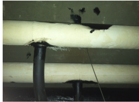
Photo 6. Asbestos-containing white block pipe insulation was observed in various locations throughout the building.
