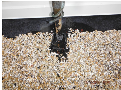
Photo 16 Black rolled-on roof flashing was observed along the perimeter and along the base of the elevator machine room on the main roof level.
