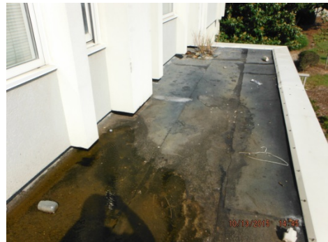
Photo 21. Black rolled-On roofing felt was observed to be associated with the front overhang roofing system.
