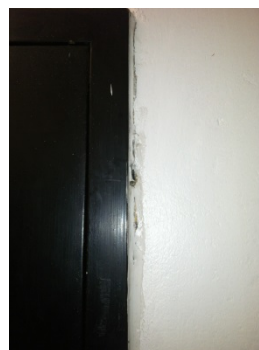
Photo 8. Asbestos-containing interior door caulking. All stairwell doors throughout the building.
