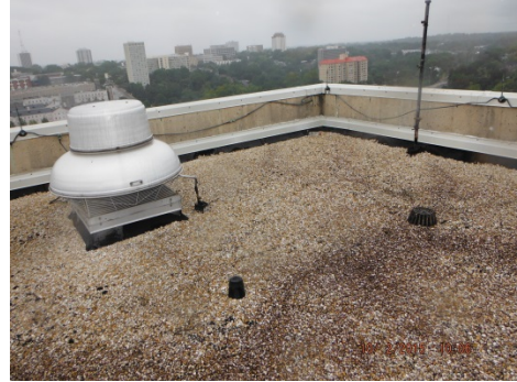
Photo 15. Black built-up roofing felt was observed on the main roof level as well as the elevator machine rooftop level.
