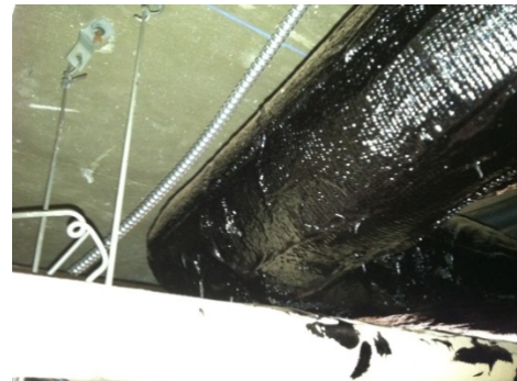
Photo 5. Asbestos-containing black mastic associated with black foam glass pipe insulation was observed in various locations throughout the building.
