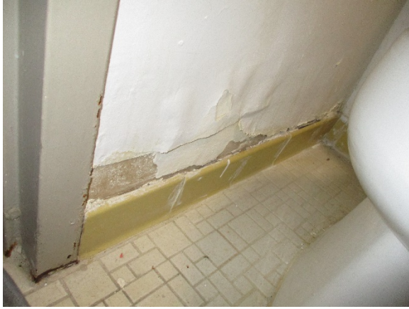
Photo 1. Damaged ACM Drywall in Room 1008.
