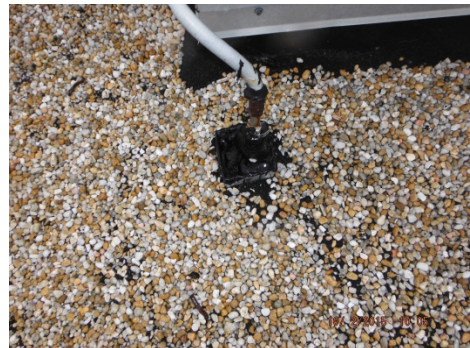
Photo 20. Black roof mastic associated with all roof penetrations on main roof level.
