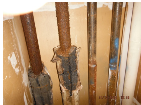
Photo 13. Asbestos-containing black mastic associated with the seams of foam glass TSI was observed throughout the building.
