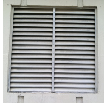
Photo 18. Gray louver caulking was observed on the side of the elevator machine room on the main roof level.
