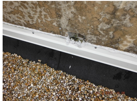
Photo 17. White roof cap caulking was observed to be associated with the perimeter of all roof levels.
