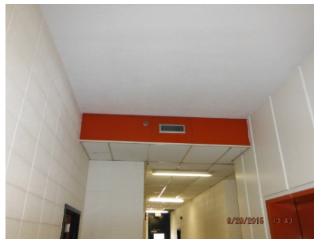
Photo 1. Asbestos-containing spray-applied ceiling texture located in various rooms of the structure.
